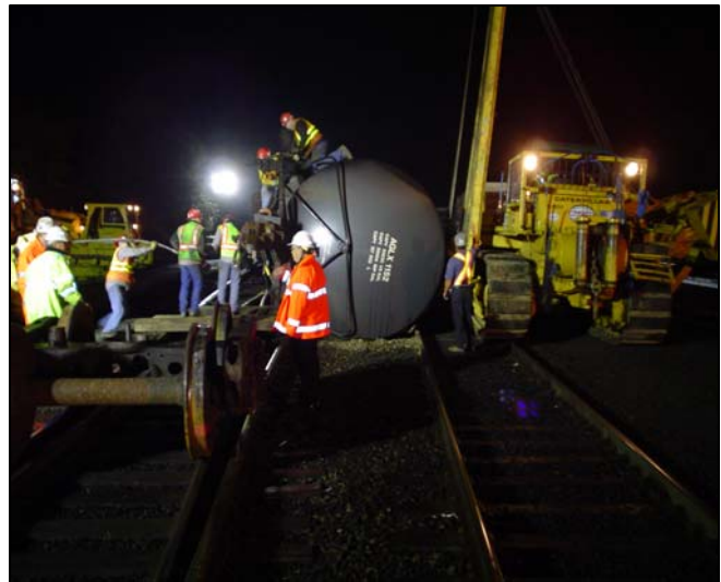
Train car derailment of highly flammable liquefied petroleum gas in Vancouver, WA (October 2006)
