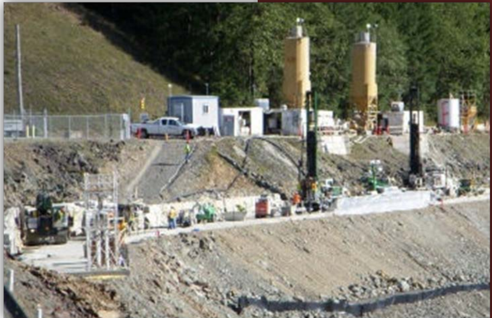
Photo (USACE): Construction for placement of grout curtain at Howard Hanson Dam.
